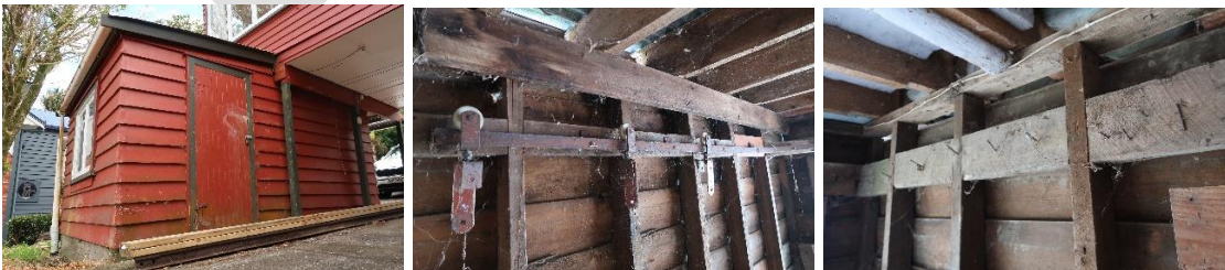
Garage, looking northwest (left), sliding door furniture (centre), and nogging with nail pegs (right)
