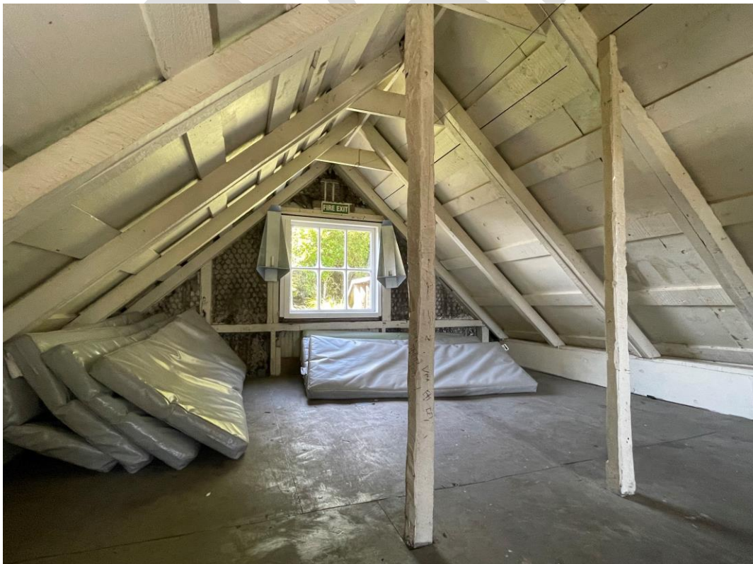
Figure 29: Loft of Field Hut looking to fire exit window on east elevation. Natalie Marshall, Heritage New Zealand, 10 March 2024.
