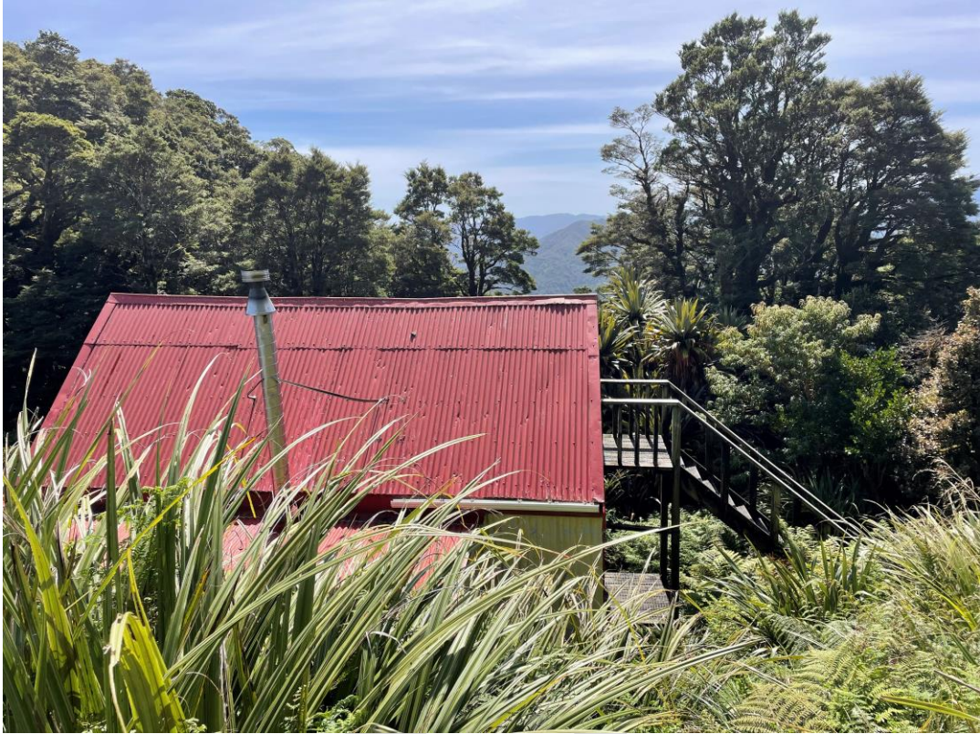
Figure 28: Field Hut, south elevation showing emergency exit from loft at rear of hut. Natalie Marshall, Heritage New Zealand, 10 March 2024.
