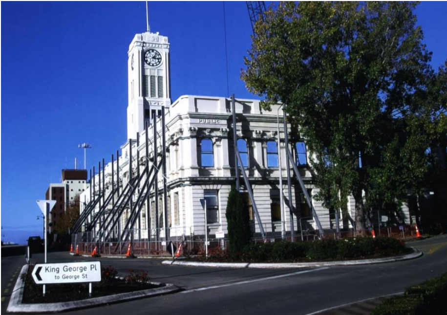
Propped façades during the redevelopment works, 13 May 2005, (photographer not known, digital image supplied to Heritage New Zealand Pouhere Taonga)
