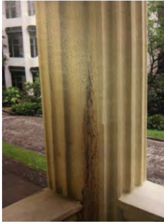
Water damage to the verandah columns as a result of the failed deck membrane above, 2009.
